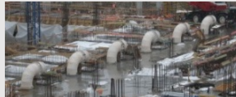
Croton Water Filtration Plant
